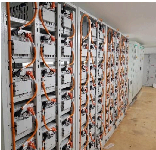
The 250kW / 600kWh BESS inside a custom-built plant room
