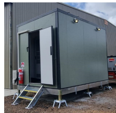
Custom Built Plant Room for the BESS
