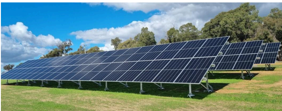
The 65kWp Ground Mount Solar Array
