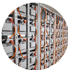
Battery Energy Storage Systems
