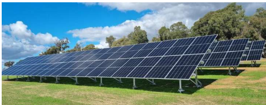
The 65kWp Ground Mount Solar Array
